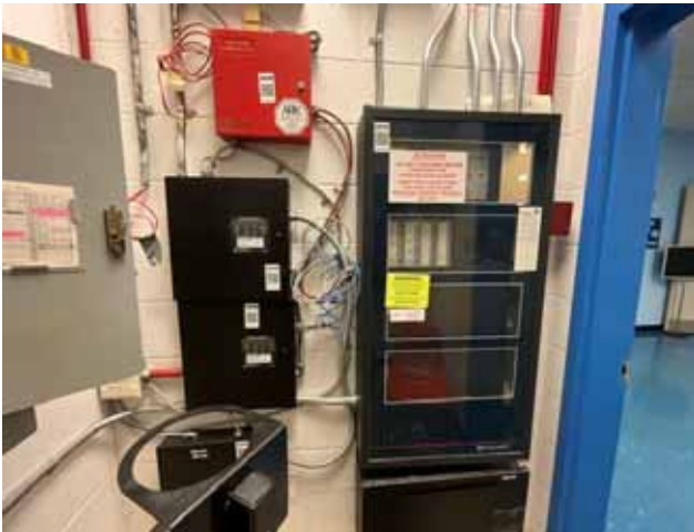
27 - FIRE ALARM PANEL
