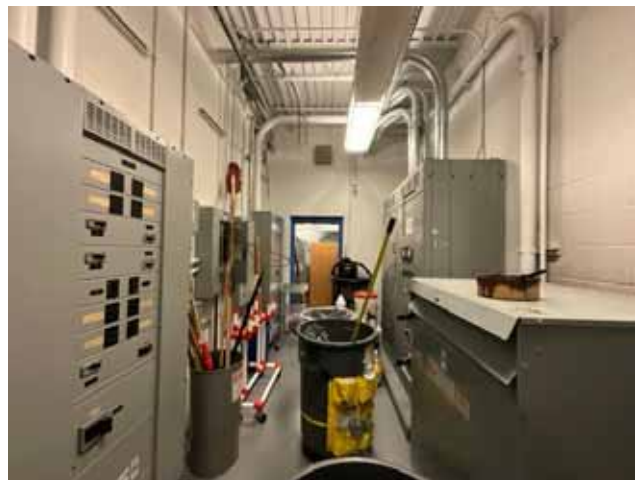
24 - MAIN ELECTRICAL ROOM
