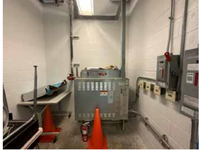
26 - ELEVATOR CONTROL ROOM
