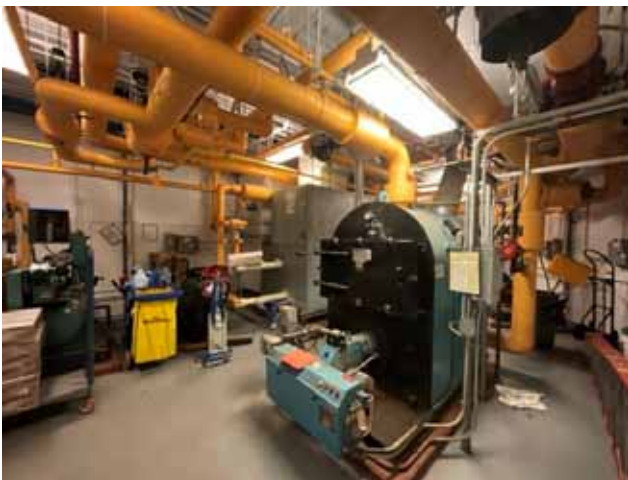
23 - MAIN MECHANICAL ROOM
