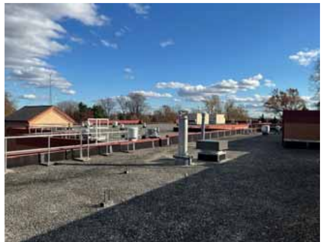
30 - ROOFTOP MECHANICAL EQUIPMENT
